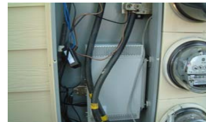
Repeater installed at meter base
